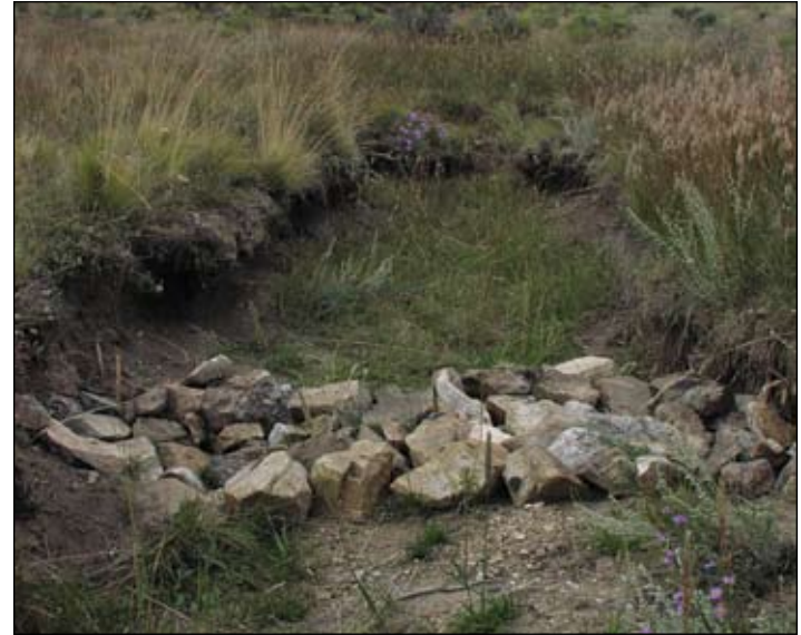
One rock dam on a side drainage of Holman Creek, Valle Vidal, Carson National Forest, New Mexico. (Photo courtesy of Tamara Gadzia.)
